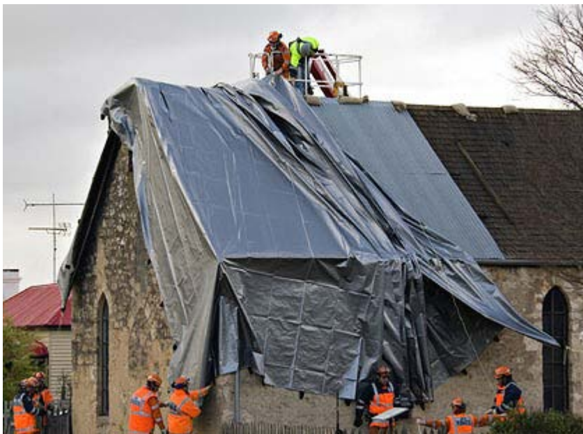
Damaged ... the Penola schoolhouse where Mary MacKillop set up her school. Photo: SMH Bruce Fraser
